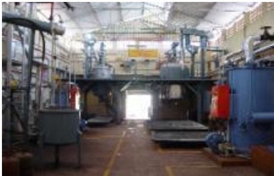
Boiler heat recovery
